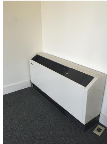
Below is a water-to-water heating unit. Units such as this one are used in buildings that have been retrofitted to be connected to the geothermal system. These units can heat fairly large room with ease.
