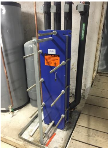
Above is an industrial heat exchanger. These units are used in buildings that were built with the geothermal system in mind. This unit is responsible for providing the energy to heat an entire building.
