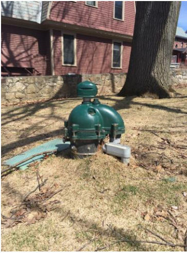
Above is production well located behind Perry Hall. This well is responsible for providing the system with the majority of its water supply.
